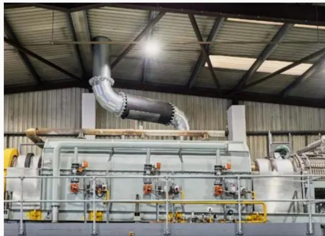
The FTU is designed to process waste plastic at a rate of 2.5 tonnes daily.
